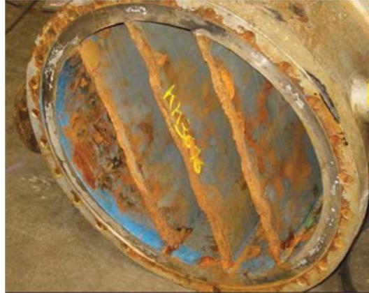
⌘ Steel coated channel in seawater service
